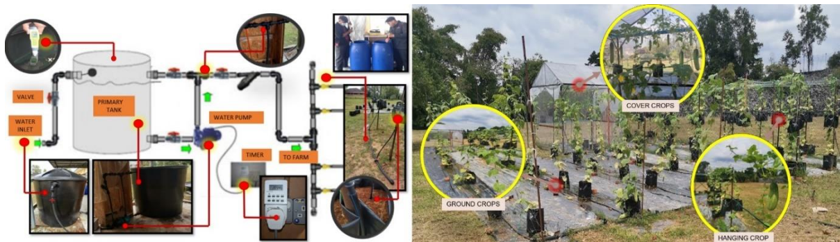
Fig. 4. Tank and Piping System Supply Water to the Farm
